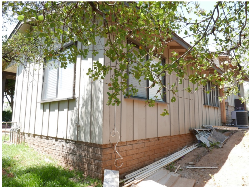
Figure 10. Northern and Eastern Façades of Guesthouse, 126 Sky Way SOURCE: Sapphos Environmental, Inc., 2017
