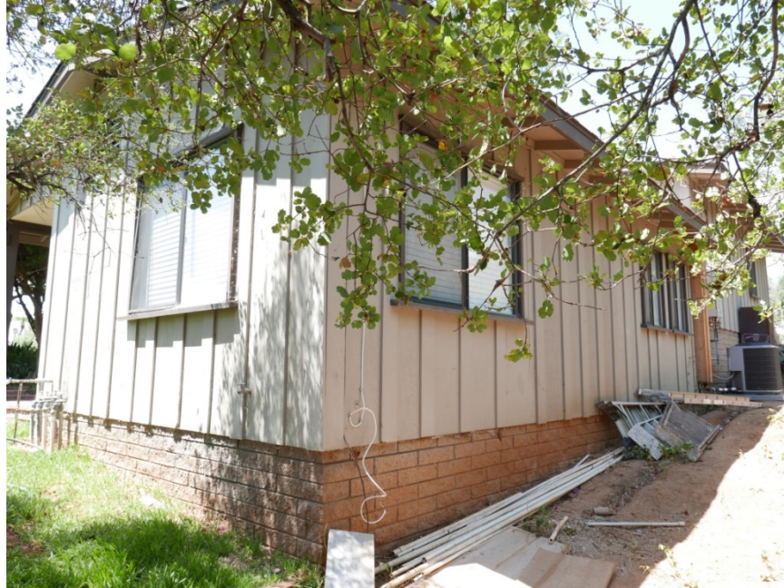
Figure 14. Northern and Eastern Façades of Guesthouse, 126 Sky Way SOURCE: Sapphos Environmental, Inc., 2017
