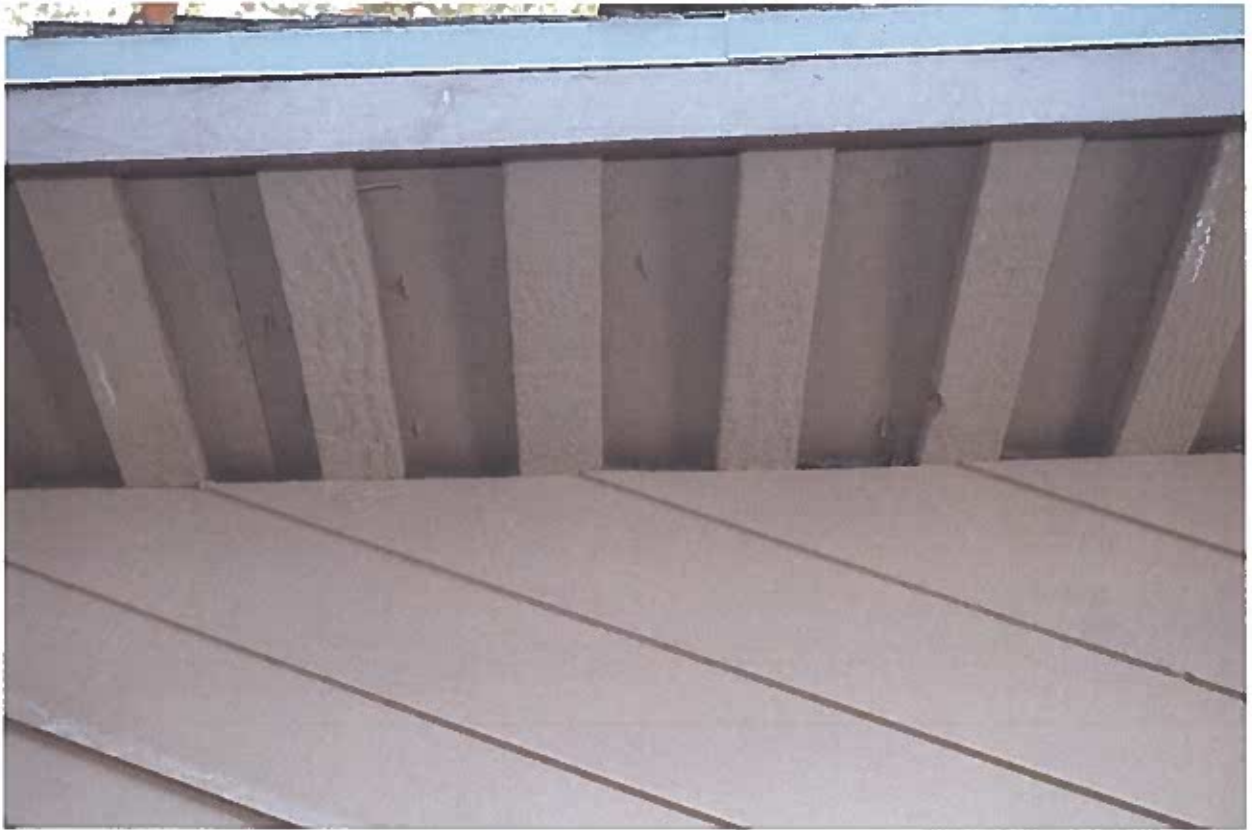
More gaps along the perimeter. Nice balcony for a rat.
