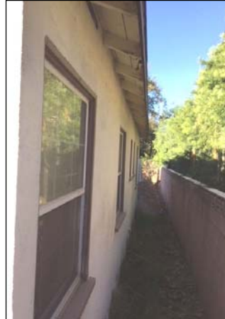
North elevation, taken from the front of the house, view to the west (2/4/18)
