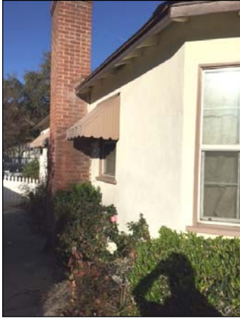
South elevation, taken from the front of the house, view to the west (2/4/18)
