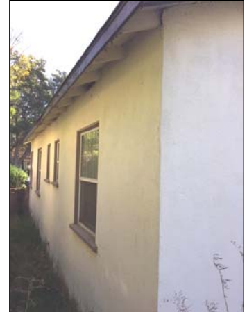
North elevation, taken from the rear of the house, view to the east (2/4/18)
