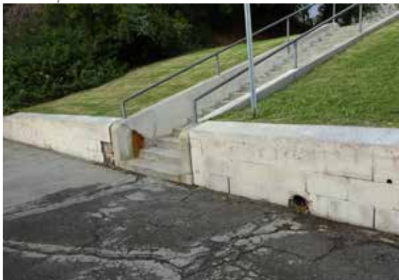
A paved perimeter path would be helpful for these users.
