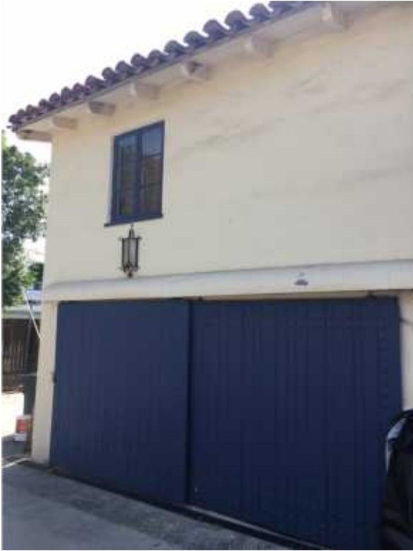
Attached two-car garage along north side of the home with original barn doors (January 2018)
