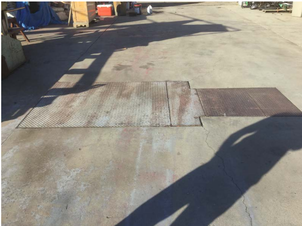
Former mechanic's pit in the steel storage yard. 126 W. Walnut Avenue, Monrovia, California 91016
