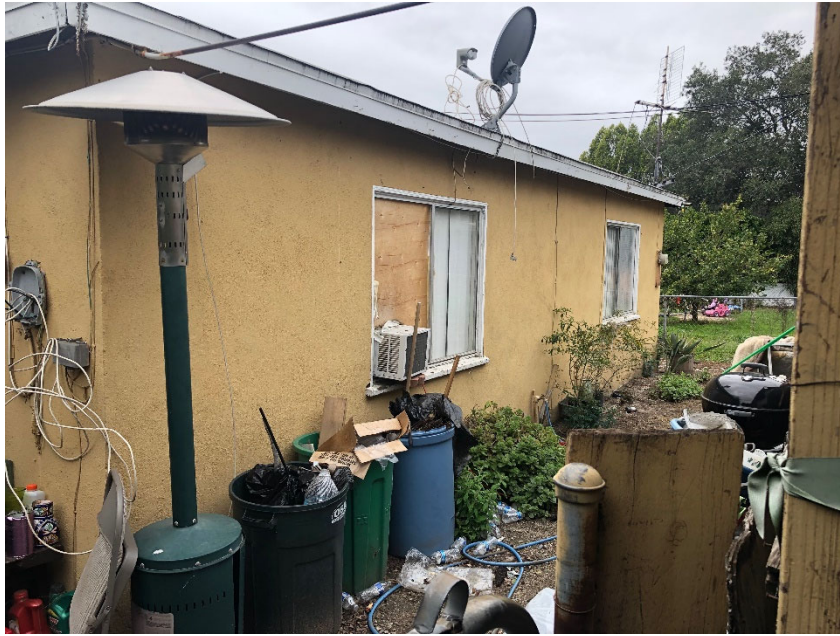
Figure 12. View of Western Façade, Rear Residence, 511 ½ E. Lemon Avenue SOURCE: Sapphos Environmental, Inc., 2019
