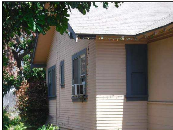
Figure 3. Photo of the front façade of 431 W Lemon Ave. The wall of the porch enclosure intersects the existing window
