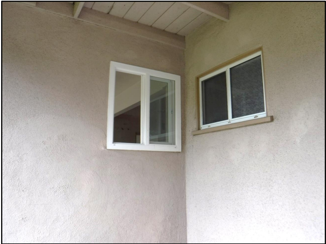
Window Detail, South and West Elevations, 1213 S. California Avenue, Monrovia, CA (NE)
