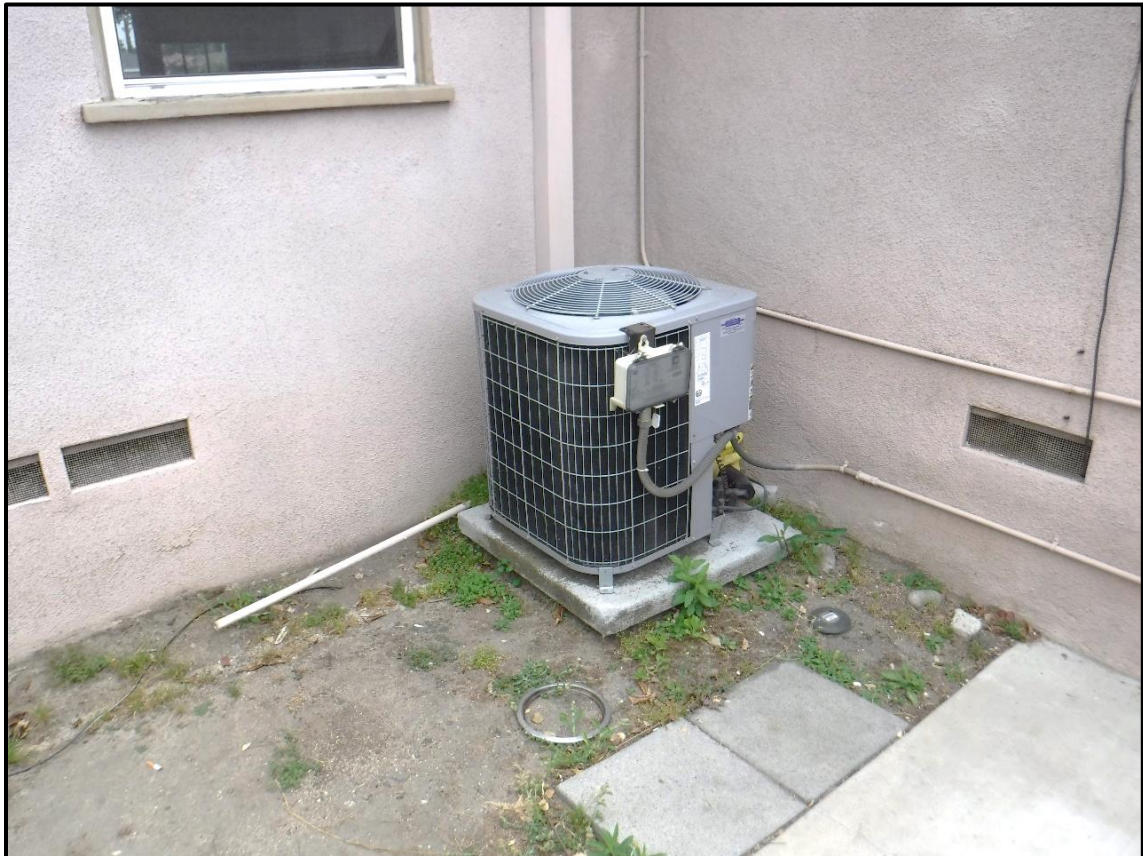
A/C Unit on West Elevation, 1213 S. California Avenue, Monrovia, CA (SW)
