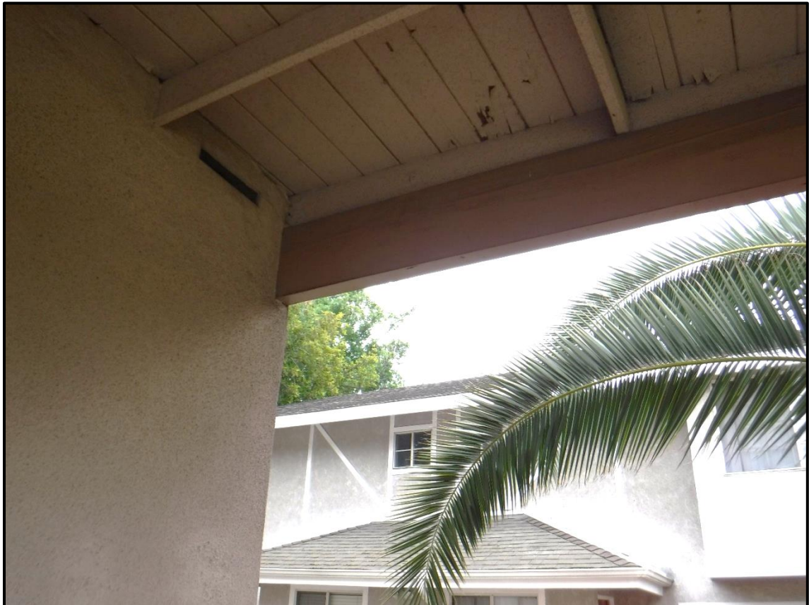
Reinforced Roof above Rear Patio, West Elevation, 1213 S. California Avenue, Monrovia, CA (SSE)
