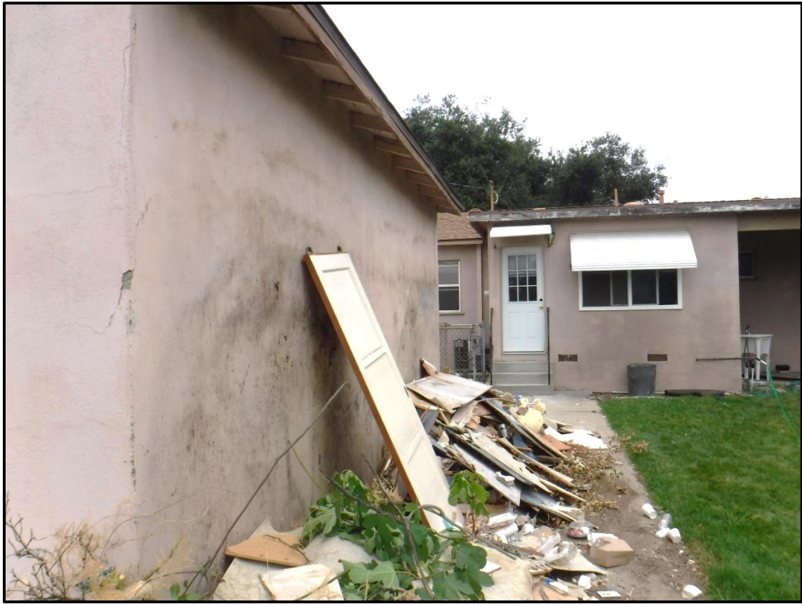
South Elevation of Garage, towards Residence, 1213 S. California Avenue, Monrovia, CA (E)
