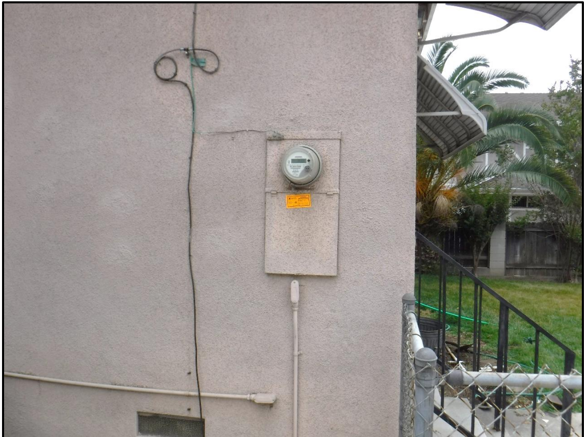
Utility Box on North Elevation, 1213 S. California Avenue, Monrovia, CA (S)
