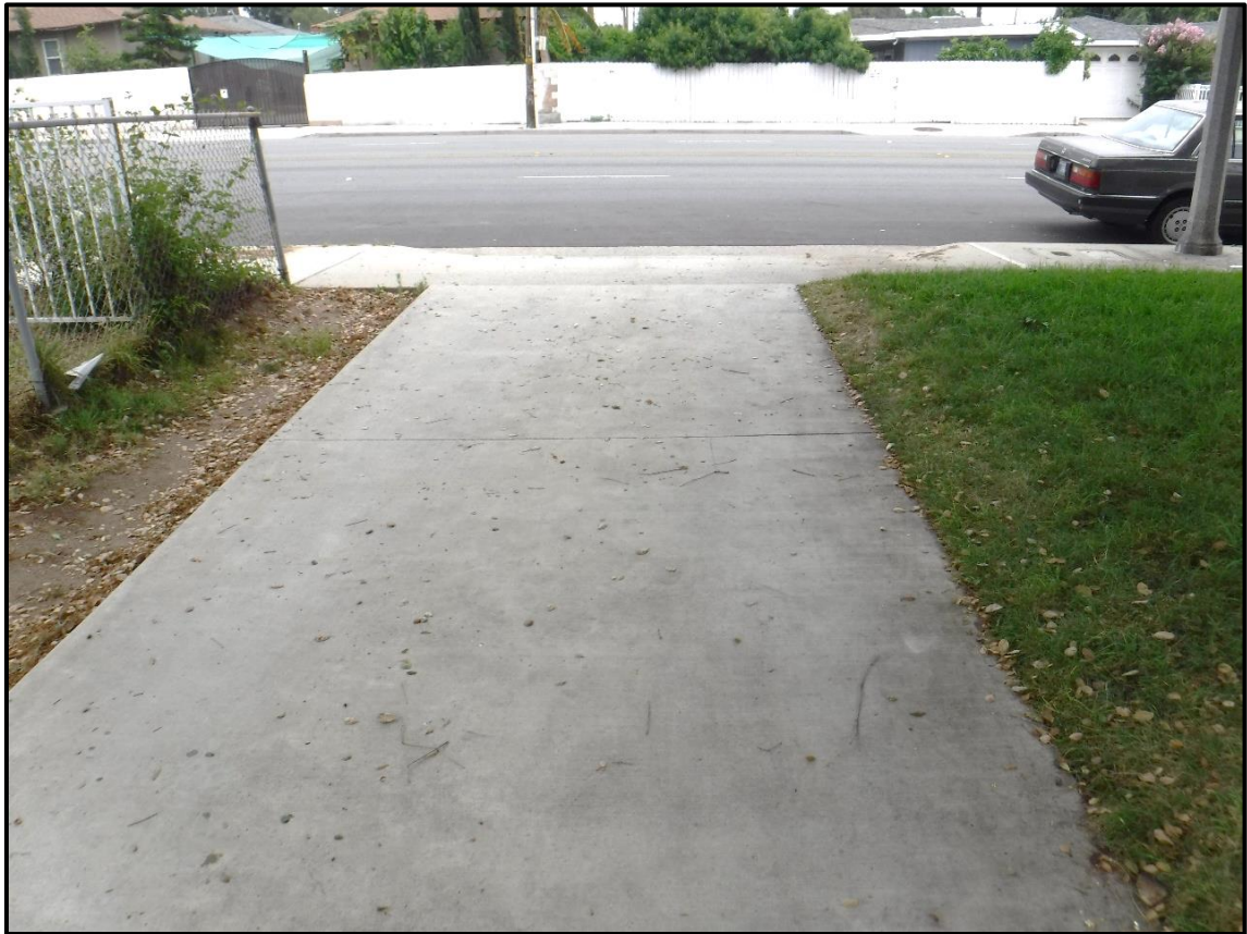
Concrete Driveway, North Side of Property, 1213 S. California Avenue, Monrovia, CA (E)
