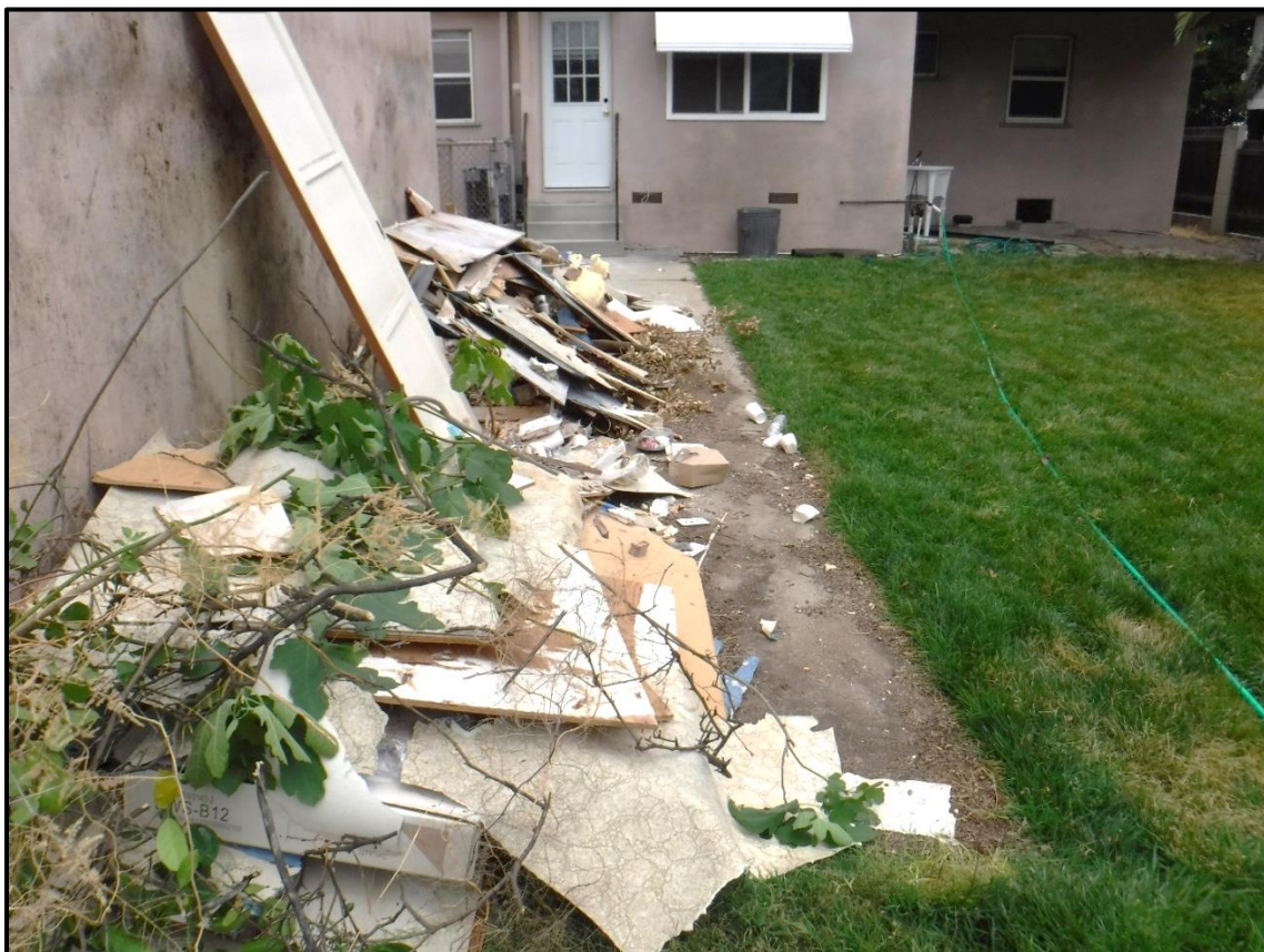
Construction Debris on South Elevation of Garage, 1213 S. California Avenue, Monrovia, CA (E)
