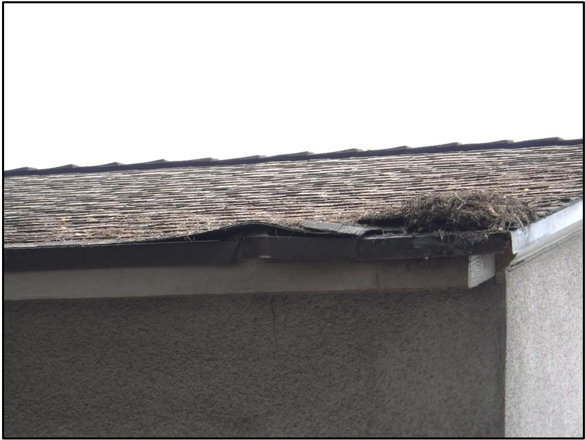
Damaged Roof, West Elevation, 1213 S. California Avenue, Monrovia, CA (WSW)
