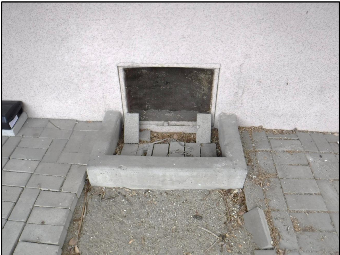
Crawl Space Entry on West Elevation, 1213 S. California Avenue, Monrovia, CA (E)
