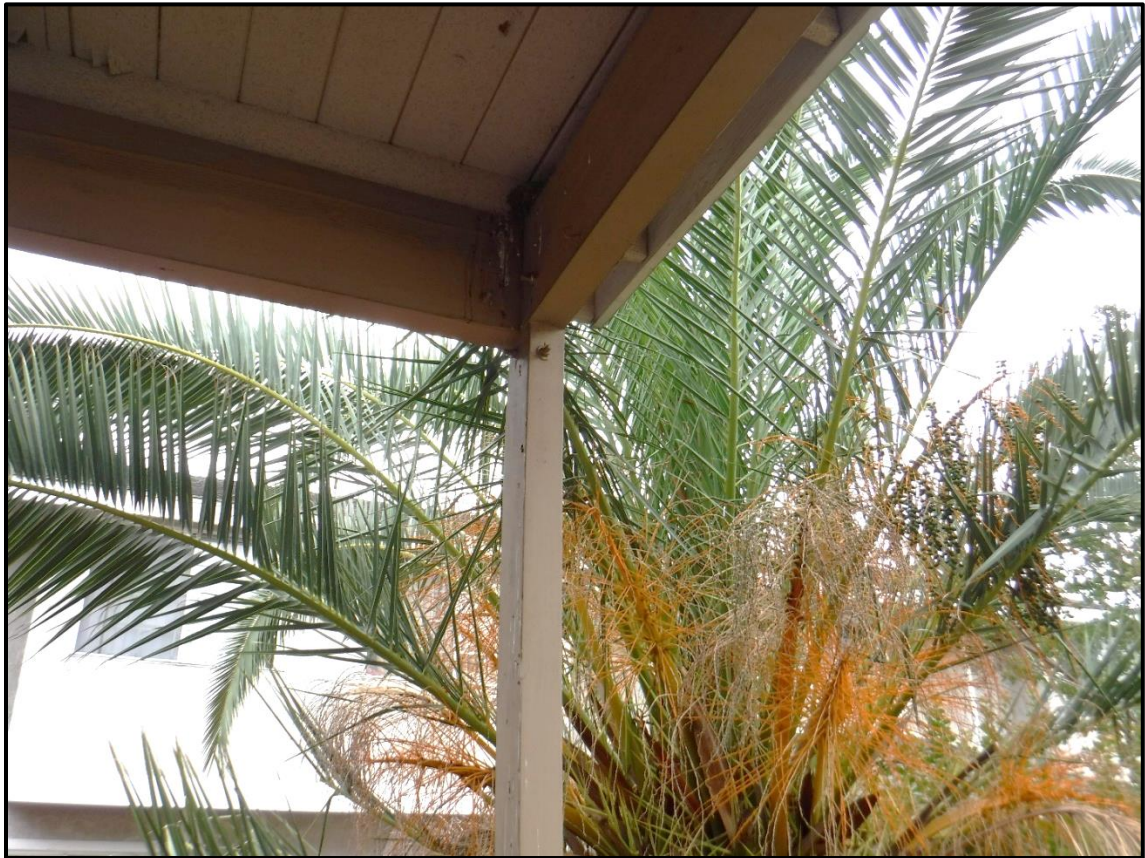
Reinforced Roof above Rear Patio, West Elevation, 1213 S. California Avenue, Monrovia, CA (SSW)
