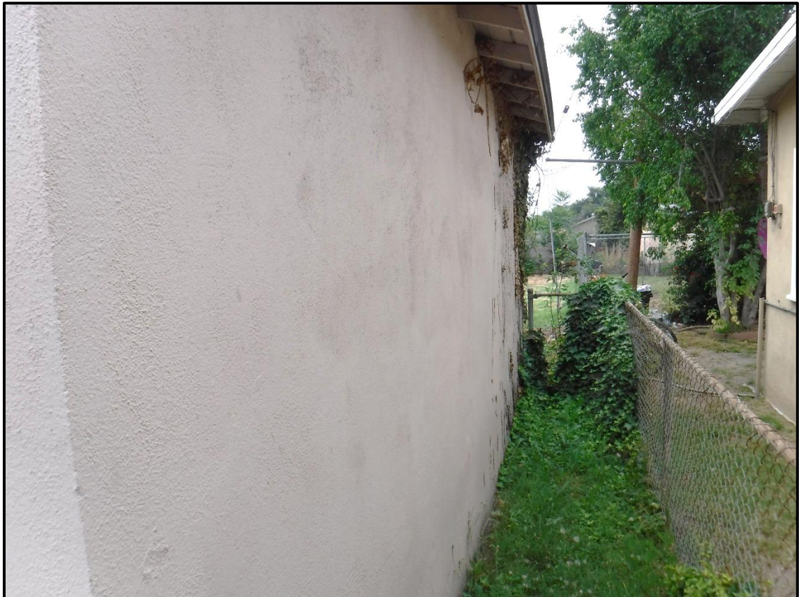
North Elevation of Garage and Property Boundary, 1213 S. California Avenue, Monrovia, CA (W)
