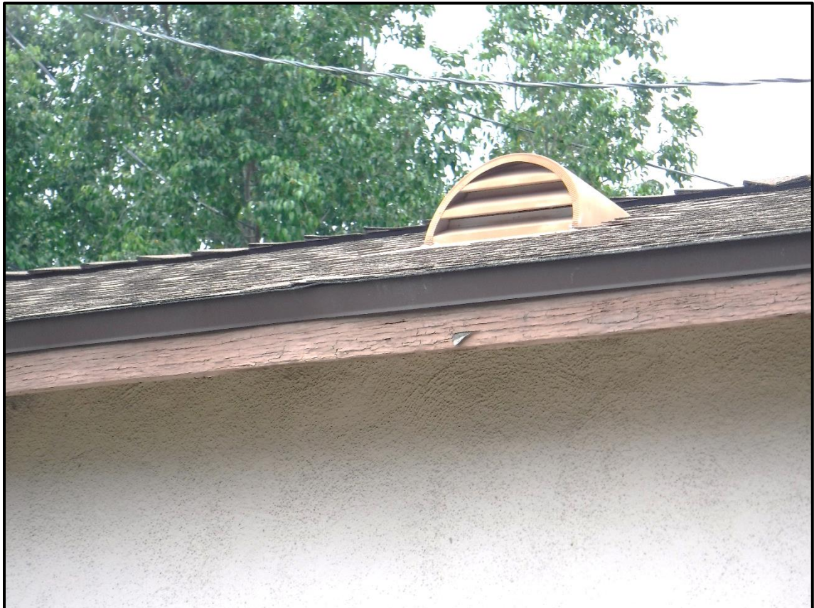
Roof Vent, South Elevation of Garage, 1213 S. California Avenue, Monrovia, CA (NW)
