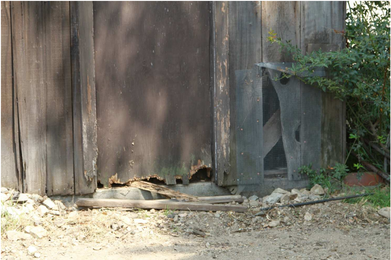
Severe decay on west side
