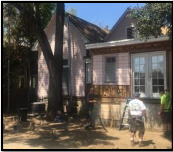
Figure 2. Photo of the rear of the house with the old deck removed. The French doors are not usable due to the sizable drop to the ground.
