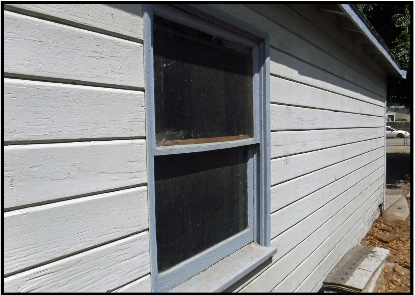
Window Detail, East Elevation of Garage, 610 W. Walnut Avenue, Monrovia, CA (NNW)
