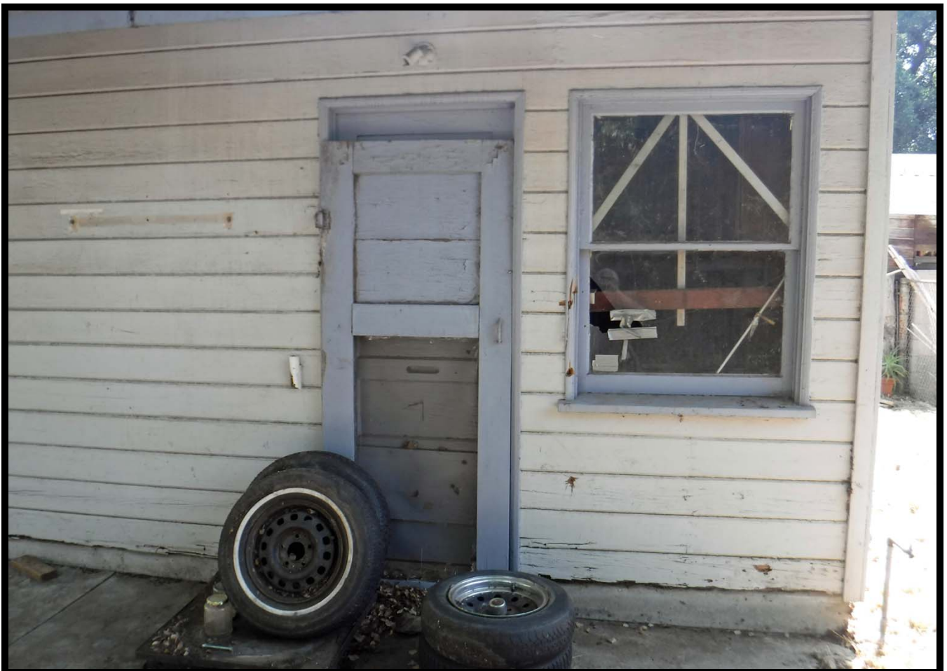
Door and Window, West Elevation of Garage, 610 W. Walnut Avenue, Monrovia, CA (E)
