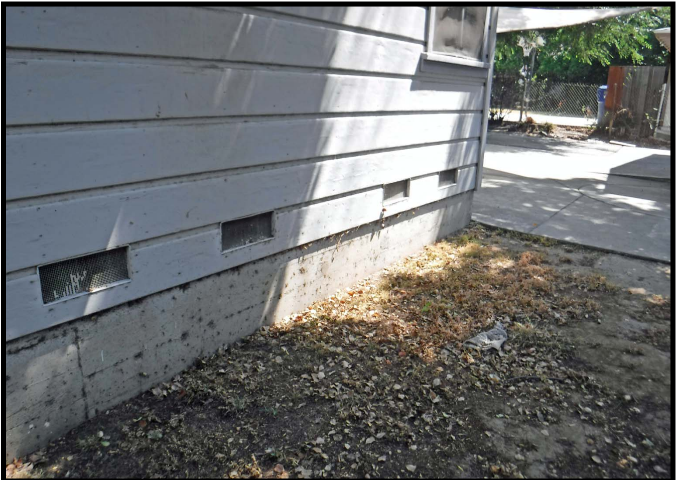
Foundation on South Elevation, 610 W. Walnut Avenue, Monrovia, CA (NE)
