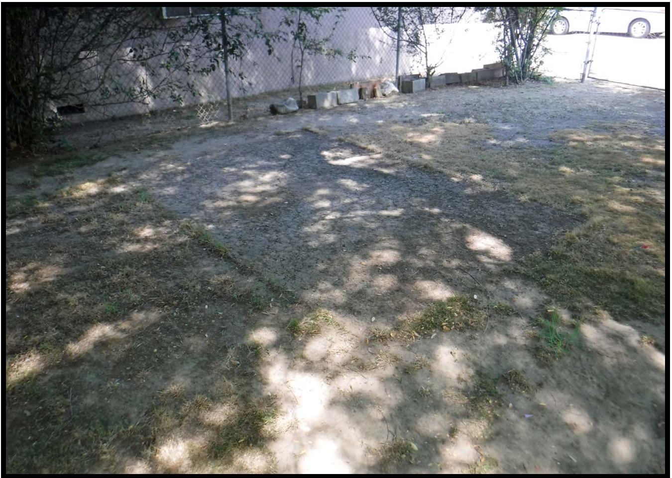
Small Structure Pad near Western Property Boundary, 610 W. Walnut Avenue, Monrovia, CA (WNW)
