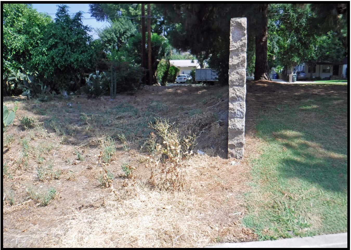
Wall Separating Properties on North Side of W. Olive Avenue, Monrovia, CA (N)
