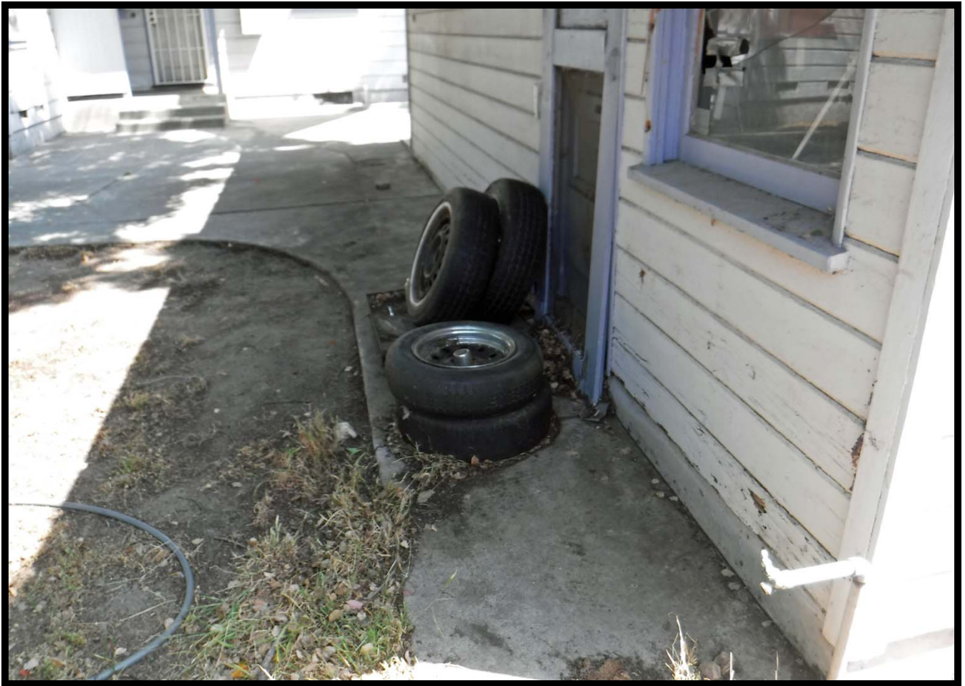
Base of West Elevation of Garage, 610 W. Walnut Avenue, Monrovia, CA (N)
