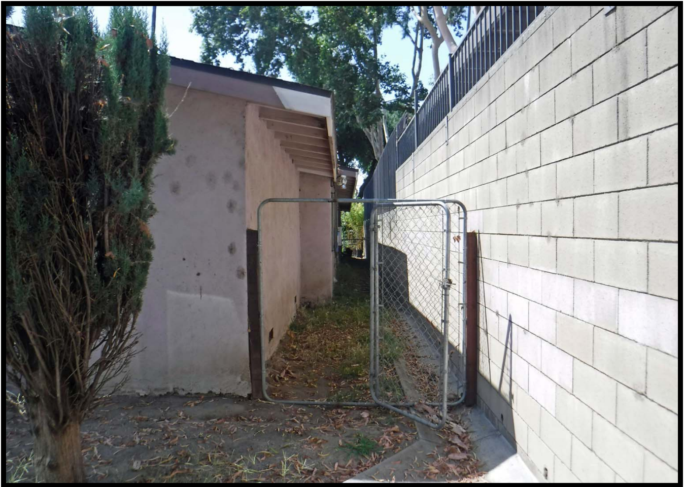
Western Property Boundary at 634 W. Olive Avenue, Units F & G, Monrovia, CA (1965; S)
