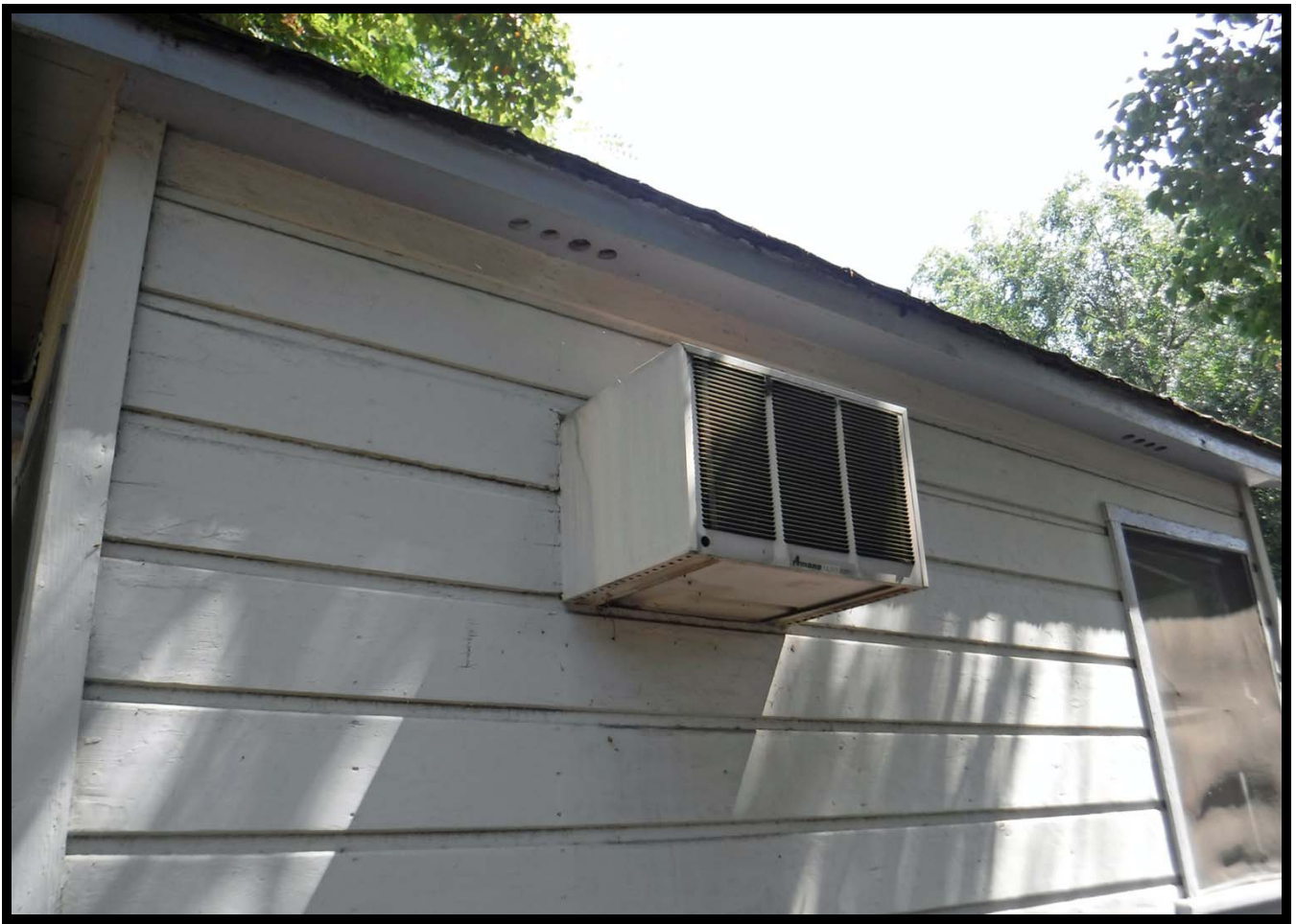
A/C Unit Mounted on South Elevation, 610 W. Walnut Avenue, Monrovia, CA (NE)
