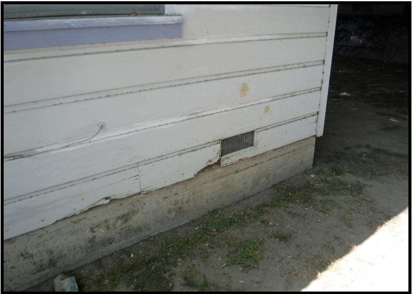
Exposed Foundation on North elevation, 610 W. Walnut Avenue, Monrovia, CA (SW)
