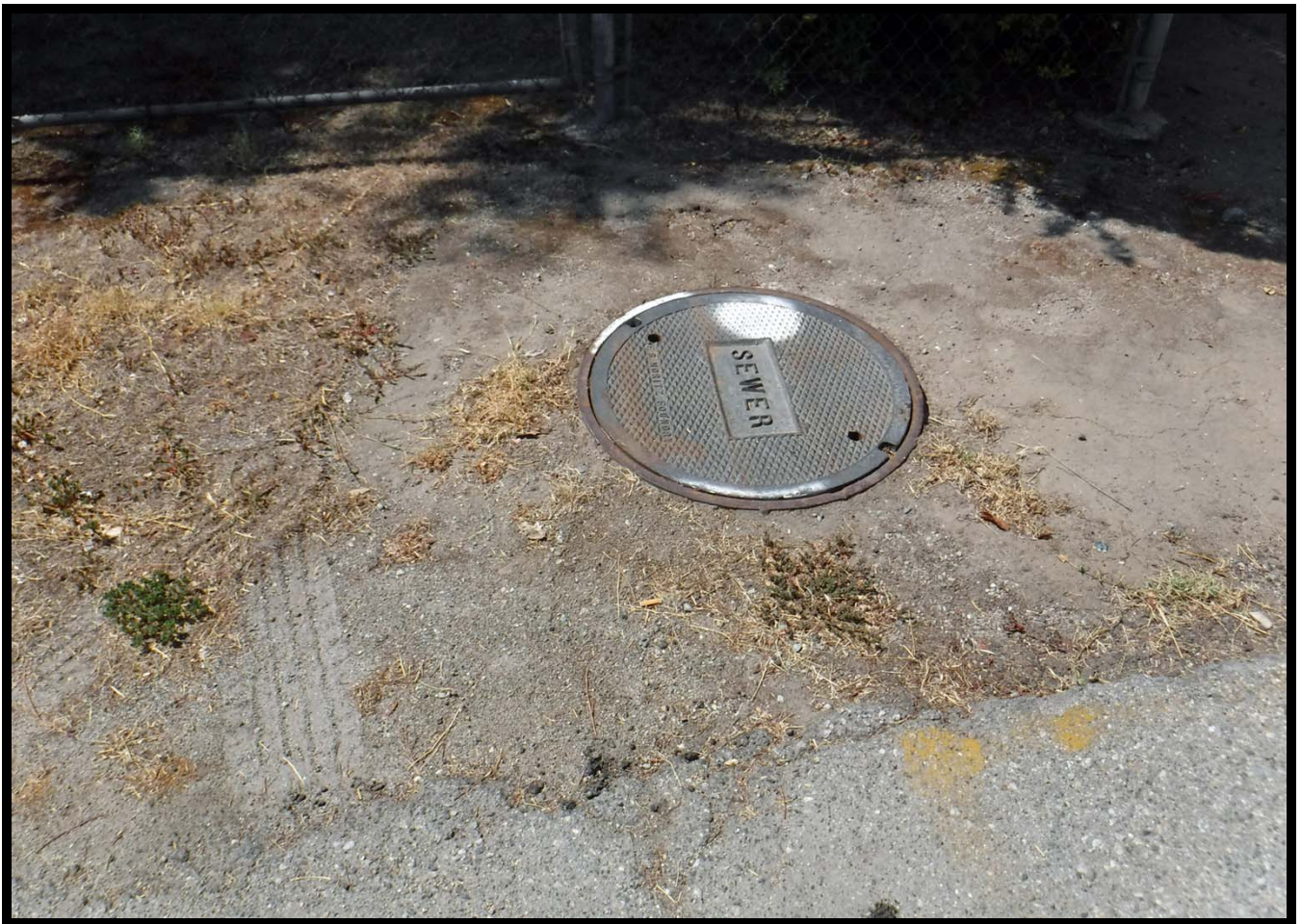
Sewer Cap on Walnut Avenue, 661 W. Walnut Avenue, Monrovia, CA (S)
