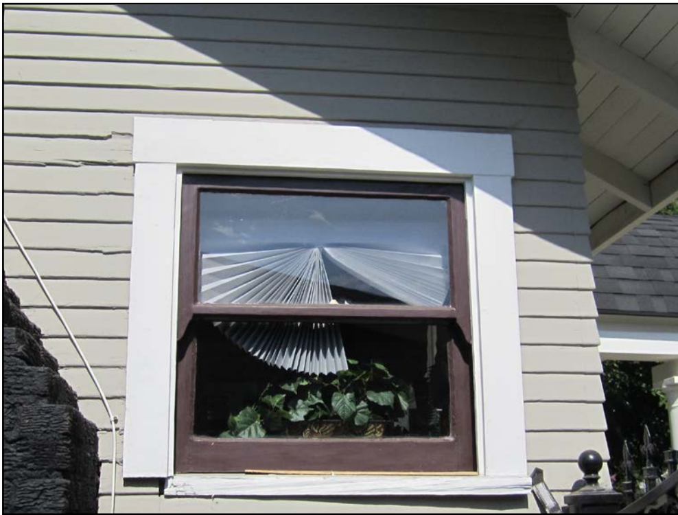
Side (East) elevation view of a single-hung window just north of the brick chimney. The window sill is partially broken and in need of replacement.
