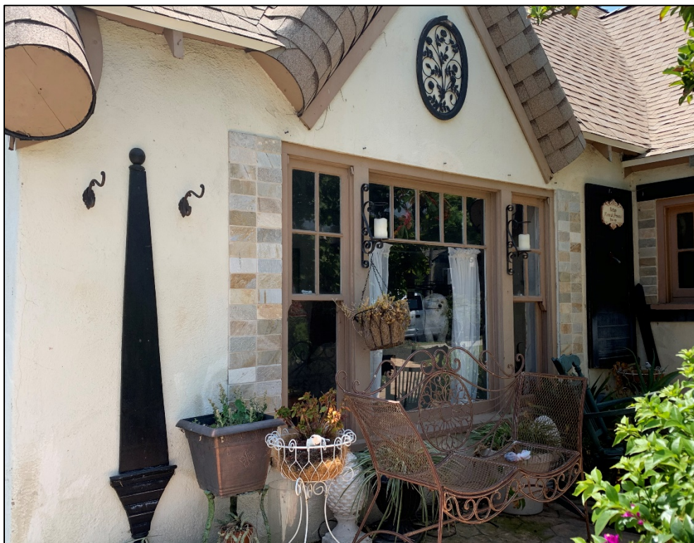
Front (North) elevation view of tripartite window located beneath the wall dormer feature. Also visible is the faux thatched roof. The brick veneer, wood, and metal features around the window are not original to the house.
