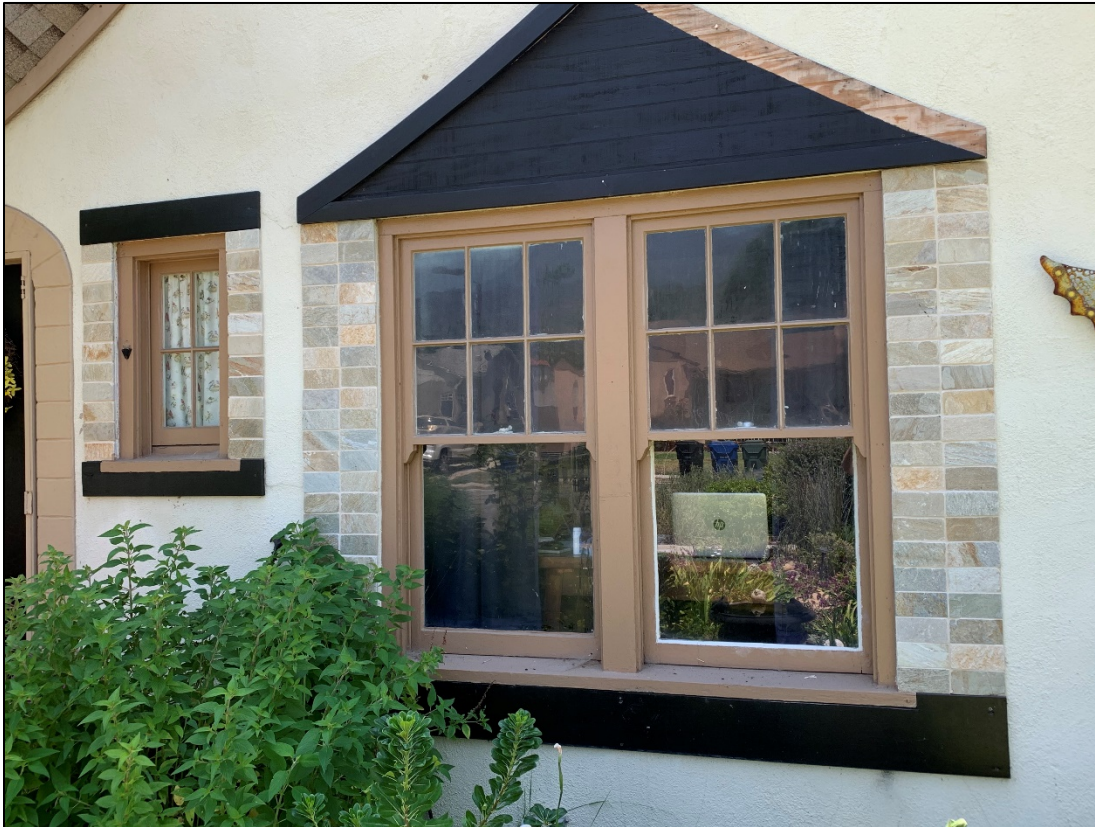
Front (North) elevation view of original multi-pane windows within the front gabled wing. The brick veneer and wood around the windows are not original to the house.
