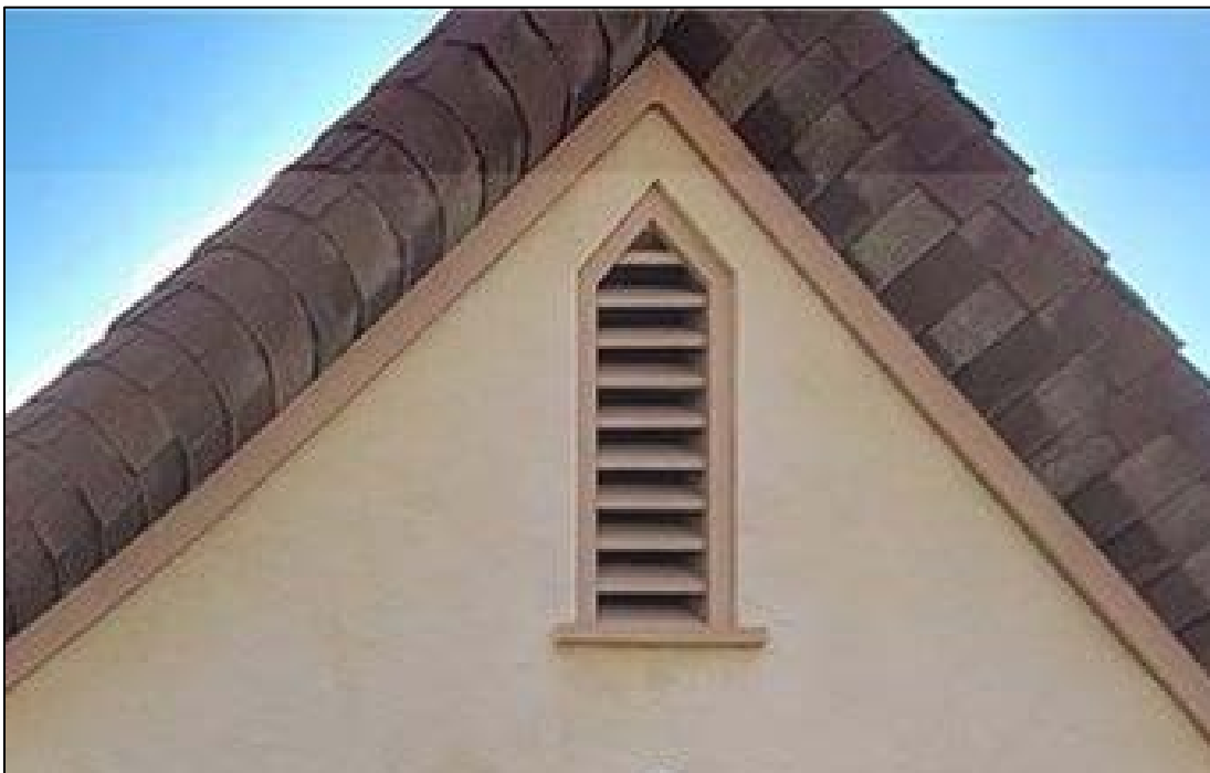
Front (North) elevation view of one of narrow attic vents with wooden louvers and Gothic style pointed arch frame.
