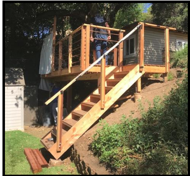
Figure 2. The deck is located off of an accessory structure and is built over the slope.
