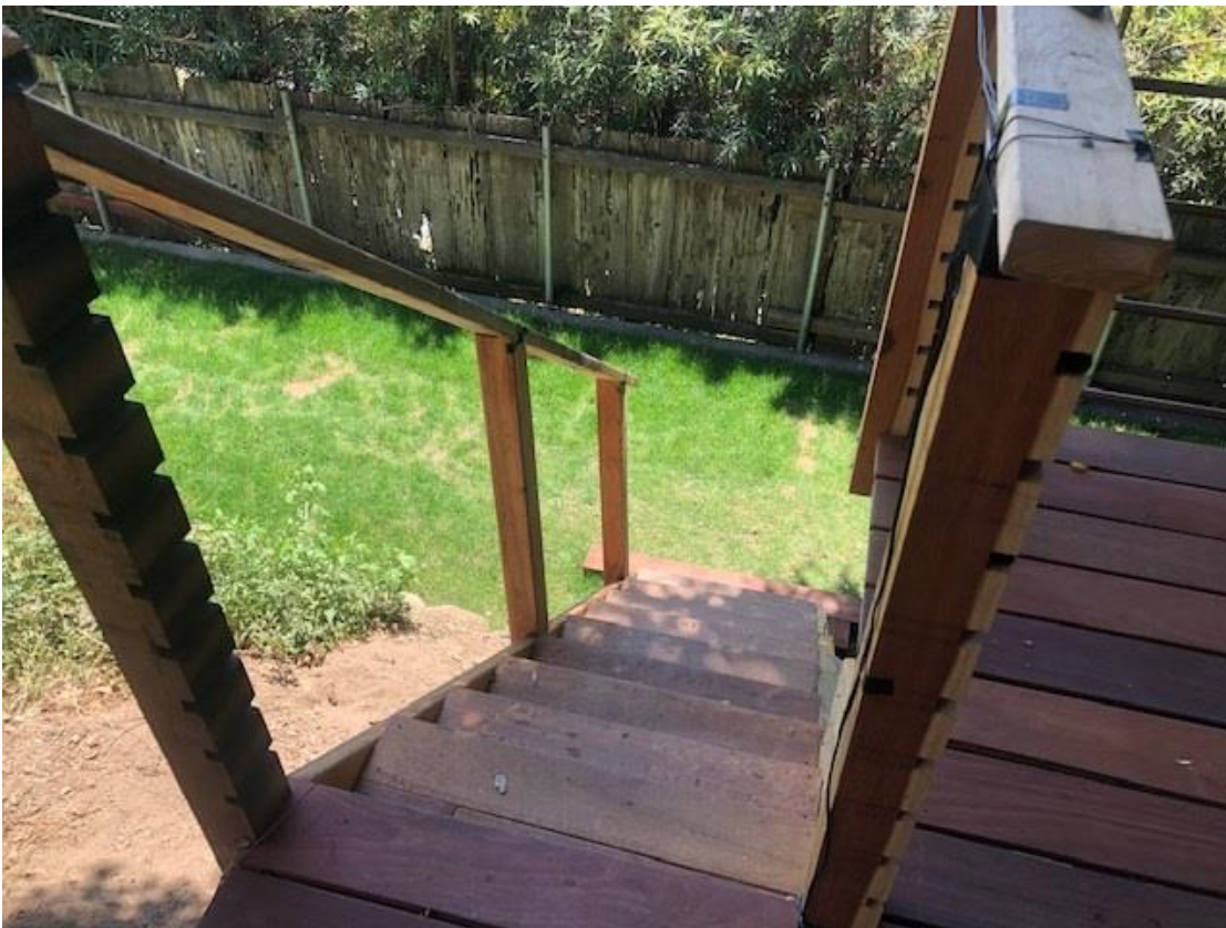
This is a view of the stairs down to the grassy area. Note that none of the railings are finished. They will be finished if I get approval.
