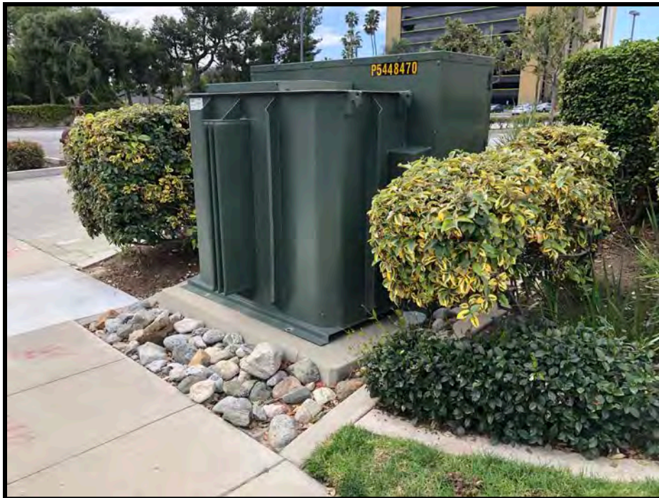
View of the pad mounted transformer adjacent to the northeastern building corner.
