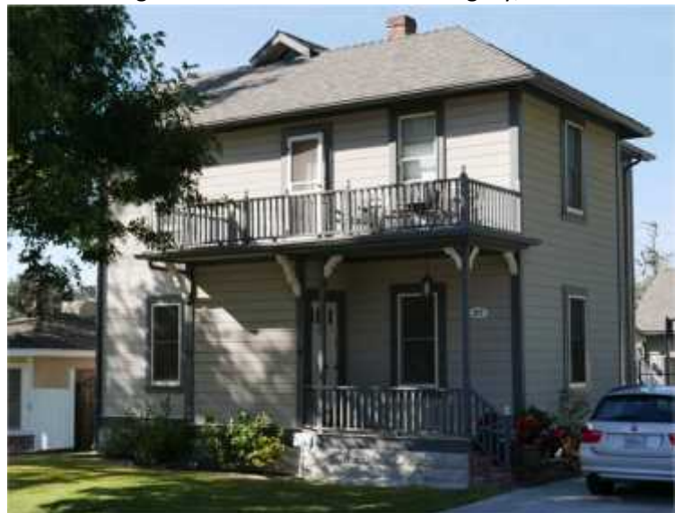
Figure 7 – Based on the architectural style, this house at 227 North Encinitas Avenue was likely built before the 1905 date in Tax Assessor records.
